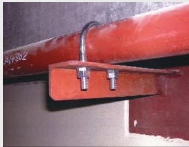
Piping in Power Plant
