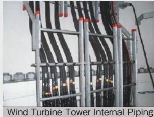
Wind Turbine Tower Internal Piping
