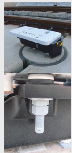
Automatic Train Stop (ATS)
